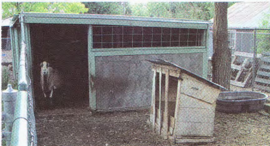
A few sheets of plywood and some 2x4s will make a perfectly suitable sheep shed.
